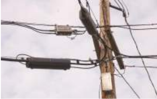
Electrical Power lines Communication
