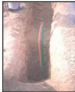
Bending Radius Not Maintained during Laying
